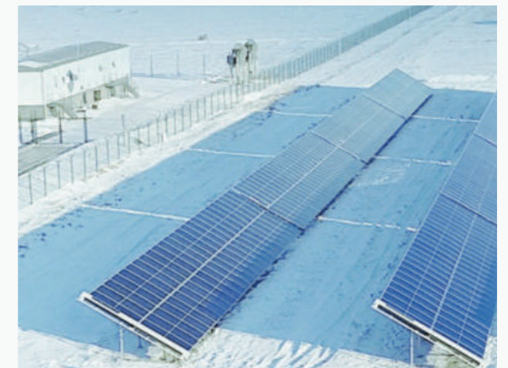
The 100MW PV power plant on the shores of Lake Balkhash
