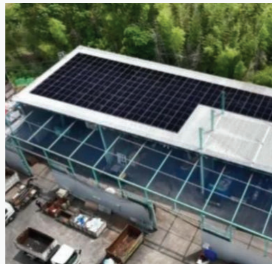
Hi-MO X6 deploying on the rooftop of the recycling factory
