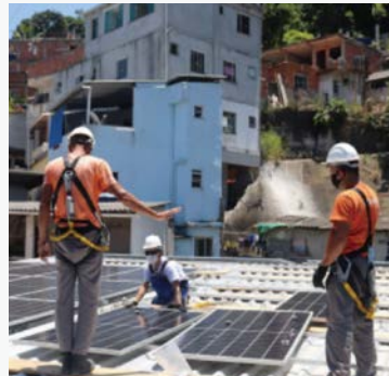
“Sun Corridor” PV Project
