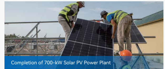
Commencement of Solar PV Power Plant at the UNHCR Regional Humanitarian Logistics Hub
