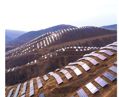
PV Power Project in Yongjing County, Gansu
